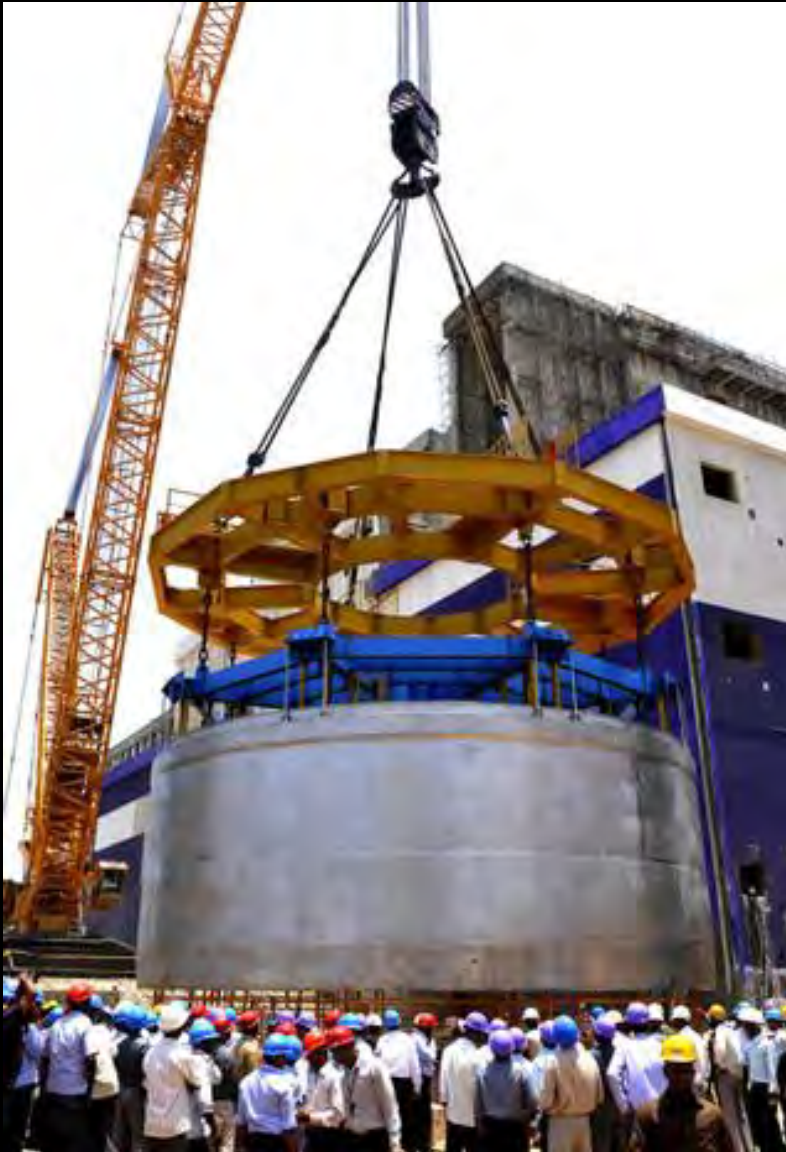
Thermal baffle being lowered into the 500 MWe Prototype Fast Breeder Reactor in India, May 2010
