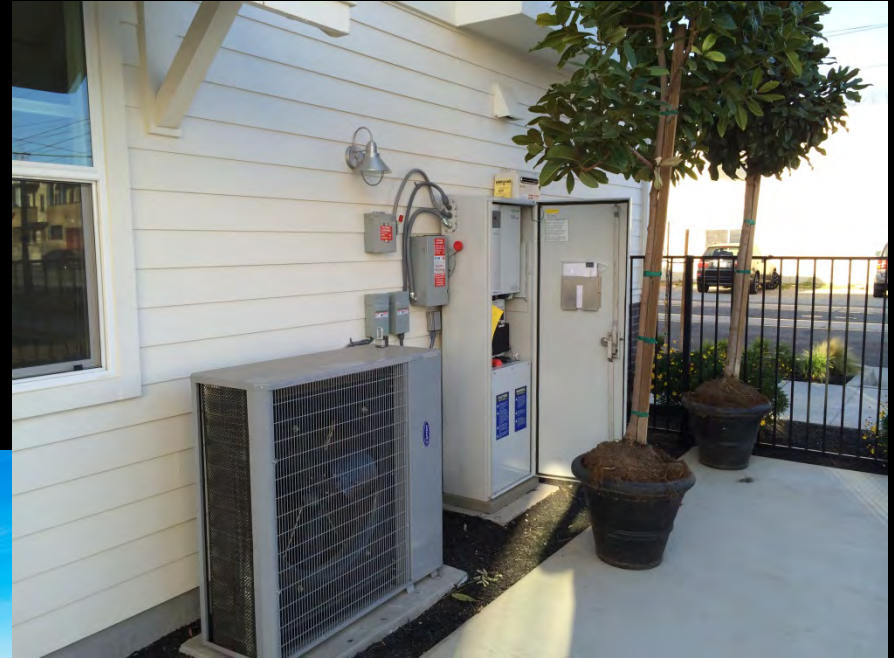
SMUD 2500 R Midtown project Sunverge Solar Integration System
